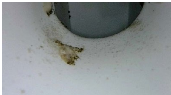
After – blockage free
